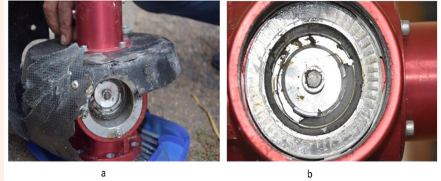
Figure 4: Aspect of the zone of the defective blade: a) as founded; b) after bearing removal.
